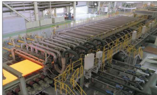
Fig 6 Combined spray and laminar cooling system at the 5m wide heavy plate mill of Baoshan Iron & Steel (Baosteel), China
